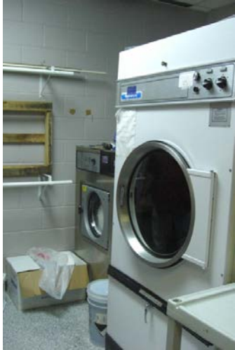
Athletics laundry, Pflugerville High School, Pflugerville ISD, Pflugerville, Texas
